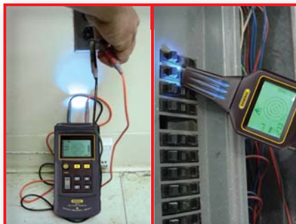
Locating a circuit breaker
